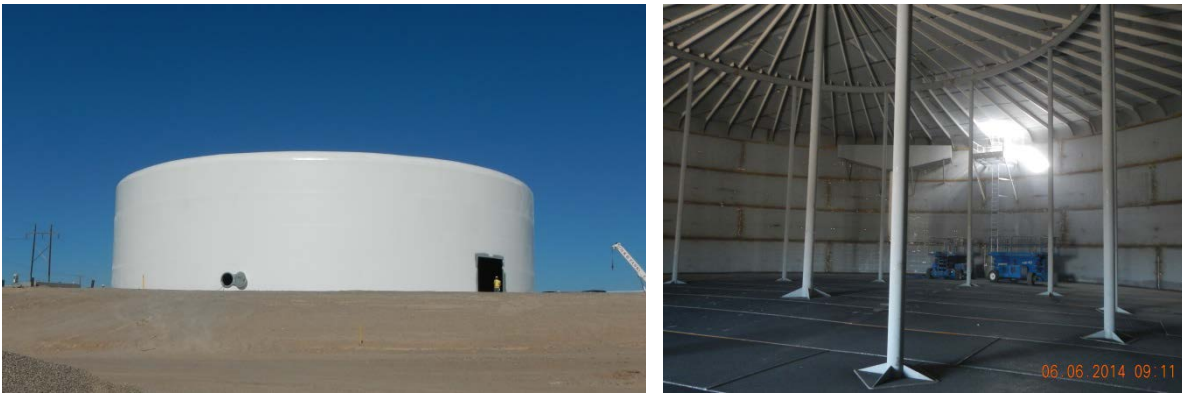
Figure 1. Construction of an 11,000 m 3 (3 million gallon) water distribution storage tank in Albuquerque, NM.
