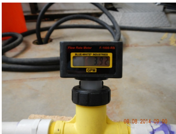
Figure 42. Flow meter used to measure fill rate during filling.
